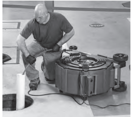
Figure 5 – Example of Extending Drain Access to within 4' (1.2 m) of Machine Cable Outlet
